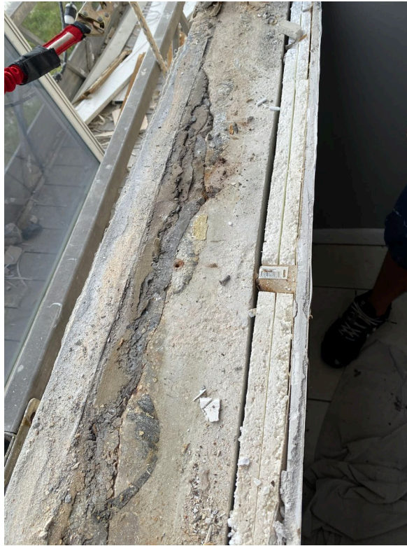
Picture 5: Crack in window sill of Unit 310
