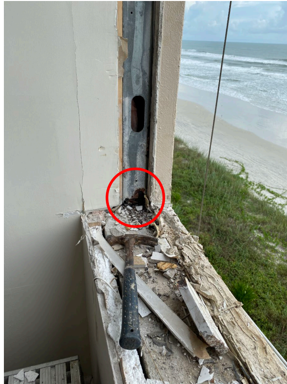
Picture 6: Metal stud corroded at bottom
