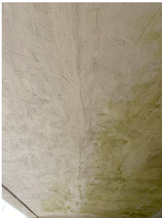
Picture 4: Crack in the bottom of the precast panel of Unit 108
